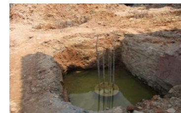
Construction of new administrative building for Jaela Division. Location:- Jaela Divisional sec. Allocation : - Rs Million. 190.7 Expenditure:- Rs Mn. 33.2
