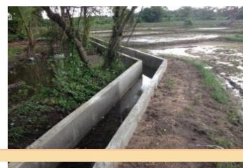
Renovation of canal at Mahawewavillege in Divulapitiya GN division Kotawehera DS division Allocations – Rs.495,000.00
