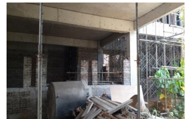
Construction of Waththala new divisional Secretariat Office building. - Waththala Divisional Secretariat Allocation - RS Million 198.8 Expenditure – Rs Million. 81
