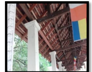
Roof renovation at Isipathanaramaya Temple, Nawinna Allocations – Rs. 1.00M Expenditure – Rs. 0.99M
