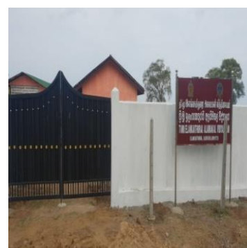
Construction of Entrance Gate at Seenaveli Athavan Vidiyalaya . Allocation - Rs. 210,000 Expenditure - Rs. 210,000
