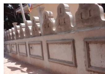
Construction of the Boundry wall at Samadarapiti Sri palithapiriwen temple, Nikaweratiya DS Allocations- Rs. 1000000.00 Expenditure – Rs. 1000000.00
