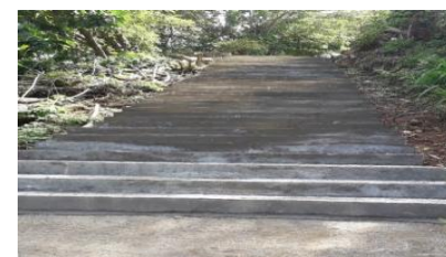
First and last part of the road next to the Mudalindarama temple road Concreted and the middle of the same road made with concrete stairway in Koggala Allocation-Rs. 1,000,000.00 Expenditure-Rs.913.896.13
