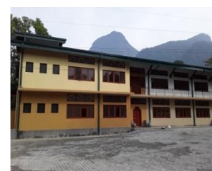
Construction of two story resting building at Sri palabaddala. Allocations - Rs.34.45M Expenditure – Rs.30.42M
