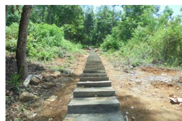
Development of the upward access road near by Viharagala Temple. Allocations-Rs.0.3M Expenditure - Rs .029M
